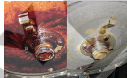
Vessel cover contaminated
